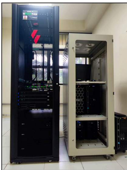
Fig. 6 Data Center do CEAMAZON.
